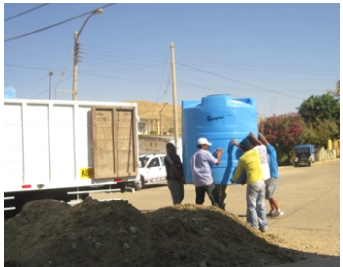
Professional installers move one of two, 2,800-liter water storage tanks from the delivery truck to the church’s chapel area for installation.
