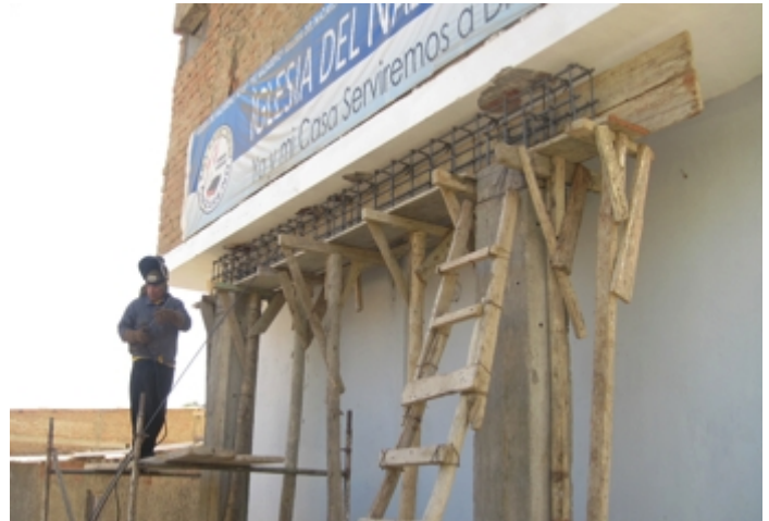
Reinforced pillars and girders were installed outside and inside the building to support the weight of a water reservoir installed above the kitchen area.
