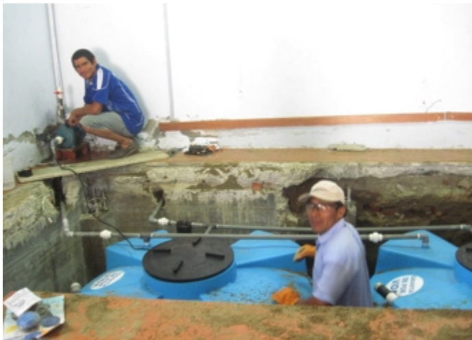
Professional installers check the operation of the water pump and look for leaks in the water storage tanks and new plumbing.
