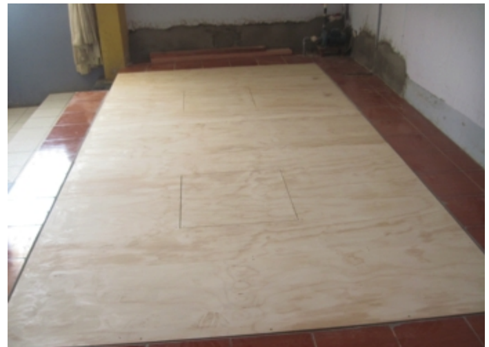
Following installation of the water storage tanks and plumbing, carpenters built a wooden support structure and cover so the area can continue to be used as a stage in the church's chapel.
